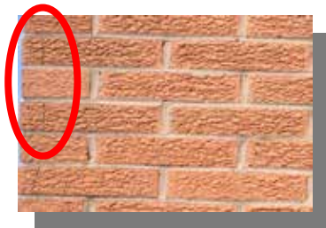
Zoom detail of crack from above photo.
